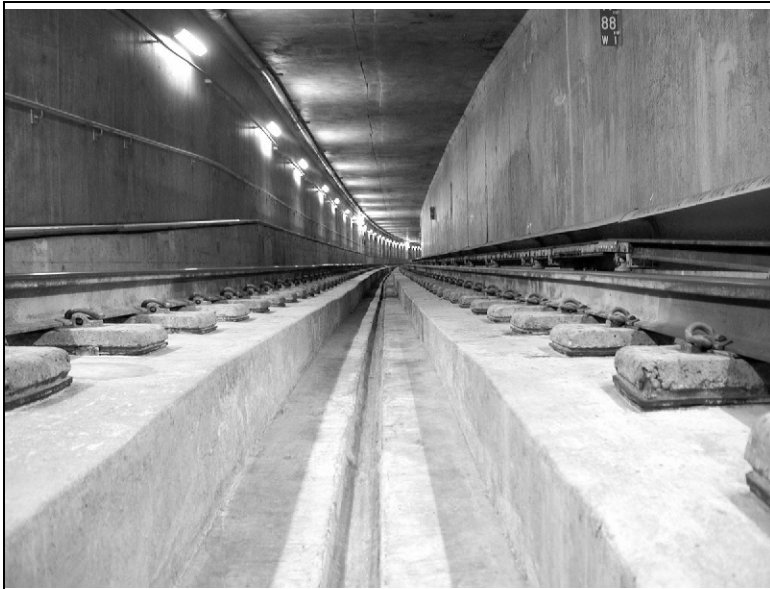
Fig. 7. Photograph of resiliently supported half ties (LVT track) in the San Francisco Airport Extension subway.
